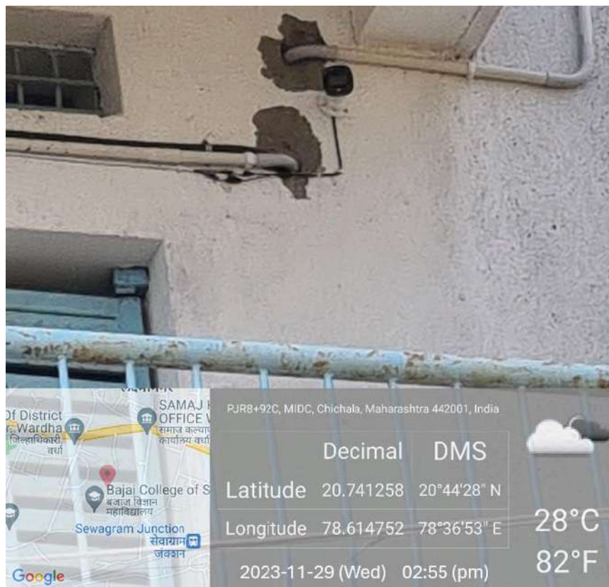
CCTV at the Girls Hostel, Bajaj College of Science Campus, Wardha.
