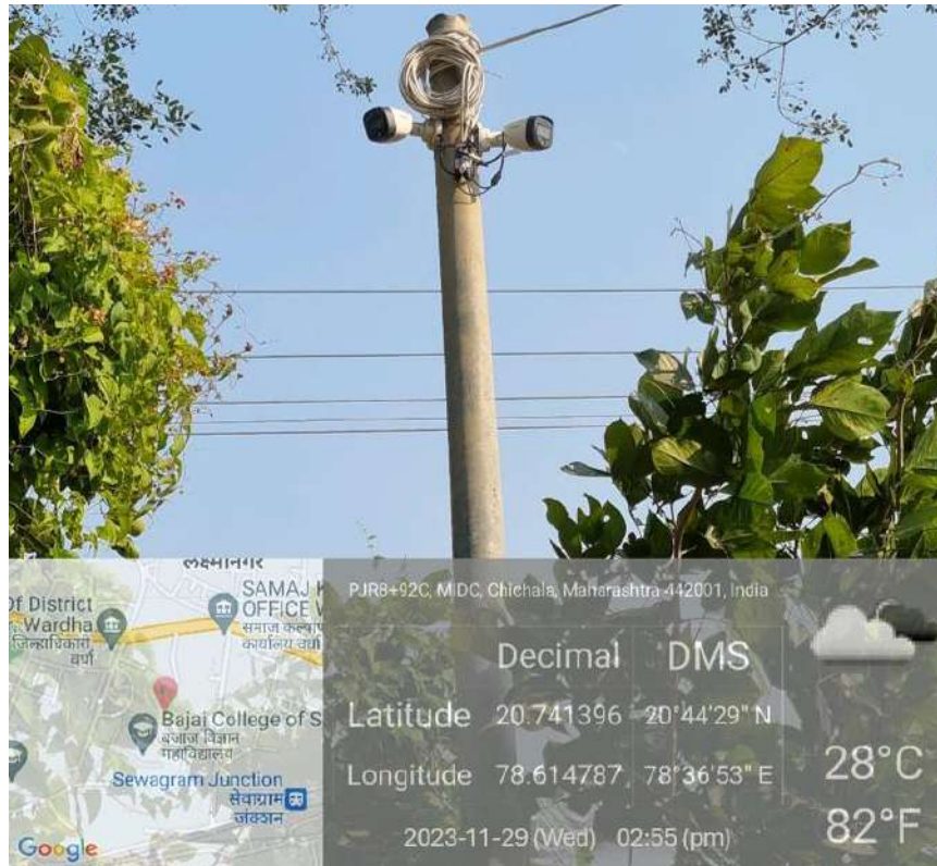
CCTV at the Girls Hostel, Bajaj College of Science Campus, Wardha.
