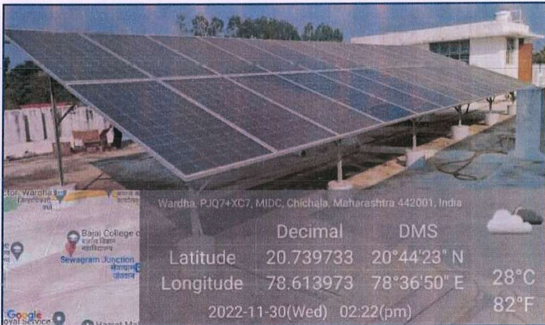
Photograph of Roof Top Solar PV Plant:
